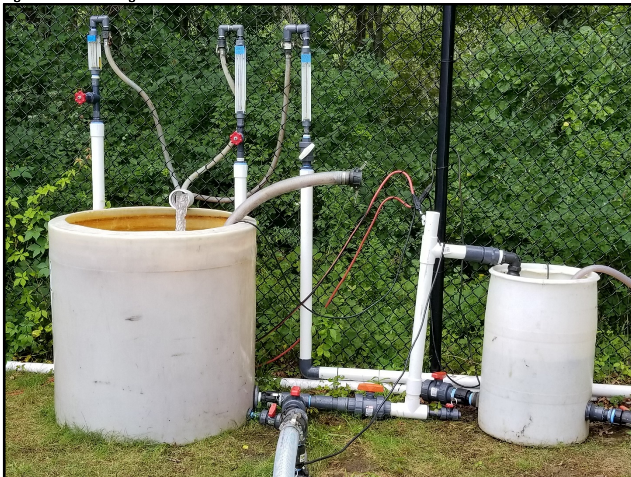
Figure 2.03: Blending Tank and Waste Tank
