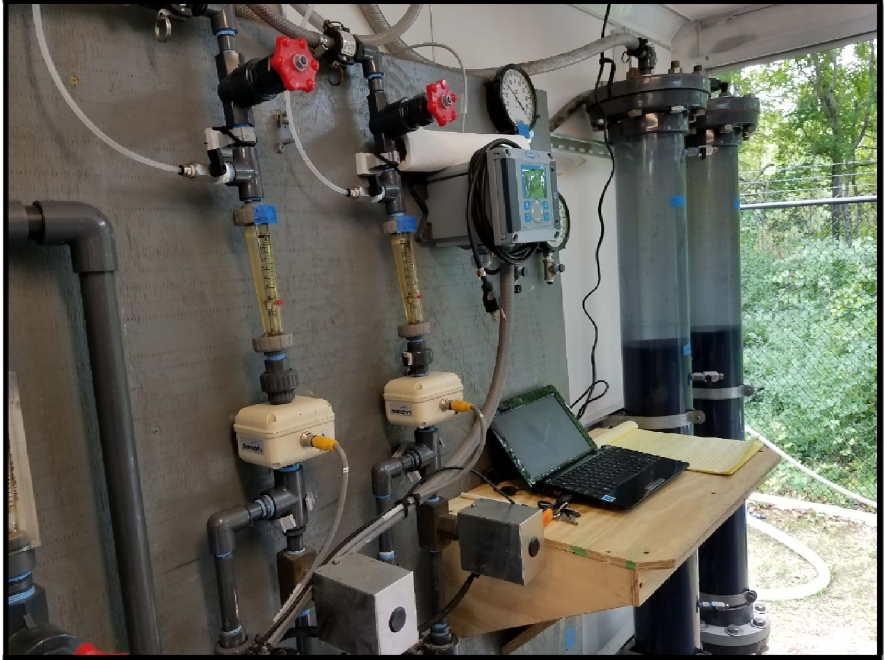
Figure 2.15: GAC Contactors and Controls
