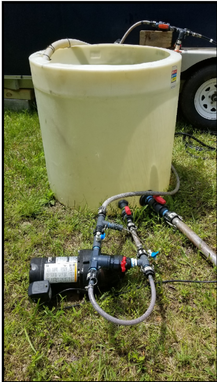
Figure 2.09: Filter Effluent Storage Tank for Backwash
