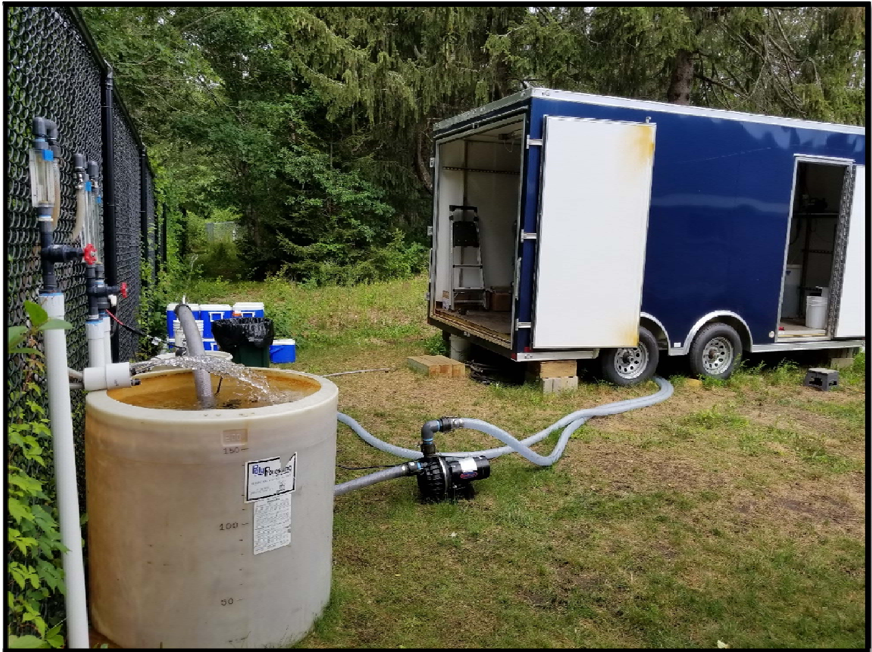
Figure 2.10: Exterior of UV/GAC Pilot Trailer at Maher Well Site
