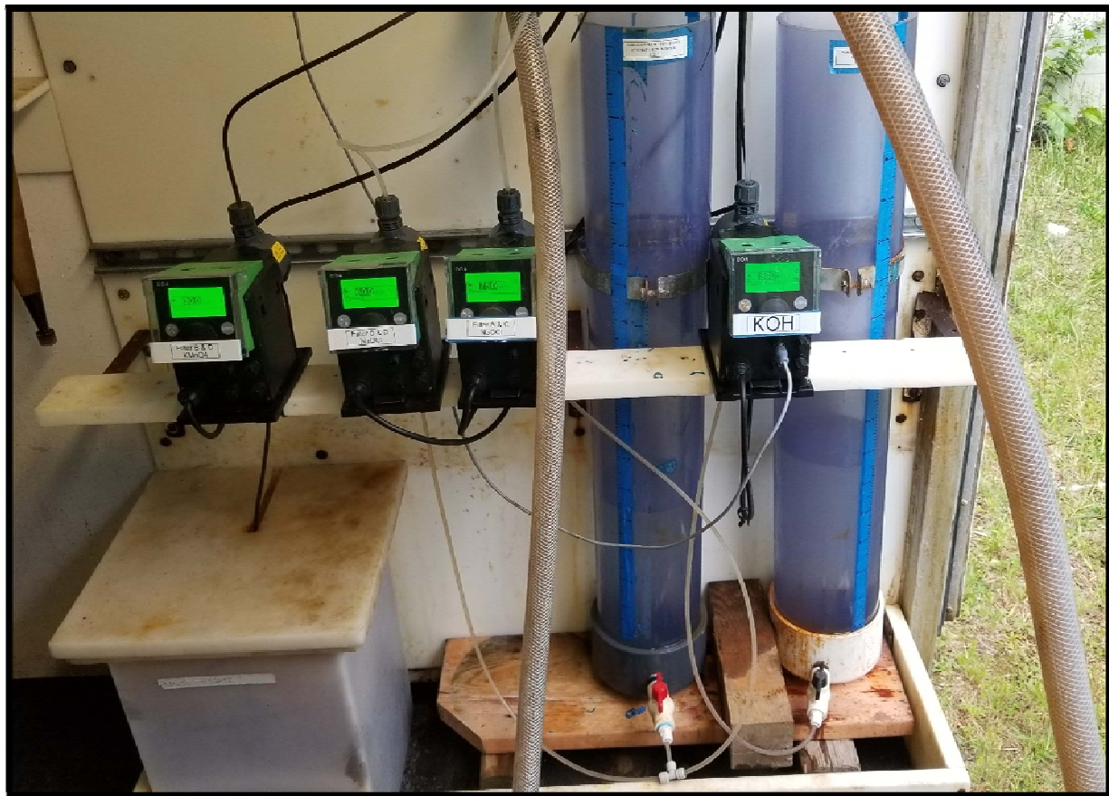
Figure 2.06: Chemical Pretreatment Pumps
