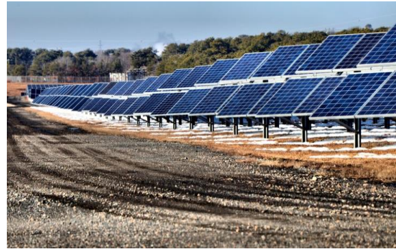
20-Acre Ground Mounted Solar Array Cape Cod Gateway Airport
