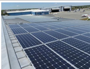
Rooftop Solar Array – Cape Air Rented Facility Cape Cod Gateway Airport
